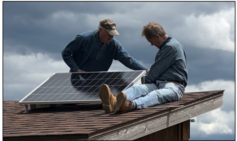
Above: Grassland Bird Trust's Peter Deming (left) works with Rob Snell of SAAS to install a solar panel on the roof of the bird blind in Fort Edward. Photo: Terry Griffin.
